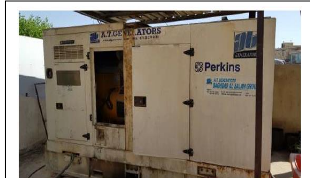
4- Turning off the Generations during their long time work
