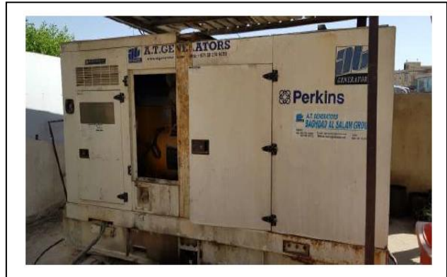
4- Turning off the Generations during their long time work
